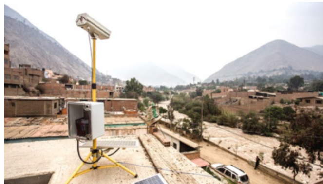
Cameras installed on a rooftop to capture pictures and collect data for the EWS in Chosica
