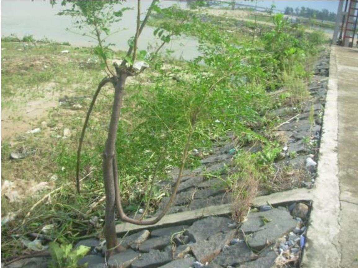
Figure 7-4: Potential impacts of wild plants growing between stones of bank protection side of flood dykes in Tuong Van
